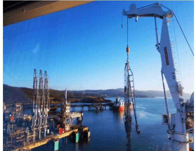
Loading arm over harbour terminal
