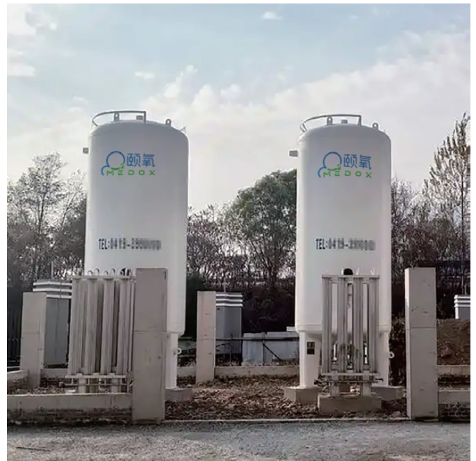
Gas Storage Tanks
